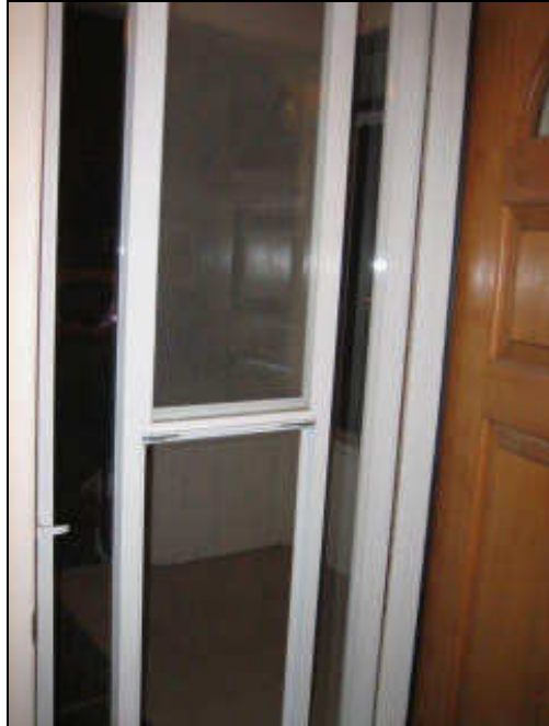
This door was damaged for the sake of art.
